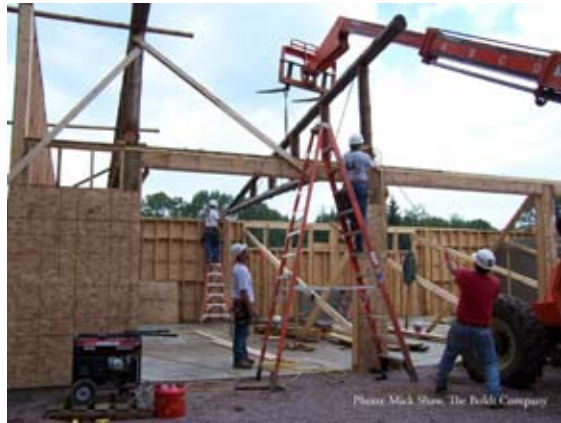
The completed trusses are carefully positioned and anchored into place with temporary supports
