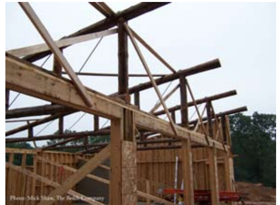
A series of five trusses will support the roof of the Axe-in-Hand Stewardship Workshop
