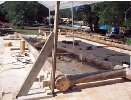
Wooden forms hold the truss at the correct angle while it is constructed
