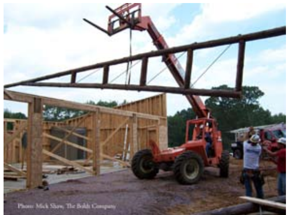
Each truss, weighing about 2,500 pounds is lifted into place with a SkyTrak forklift
