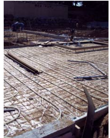
Plastic tubing will be filled with water and food-grade glycol which will circulate inside the floor to heat much of the building
