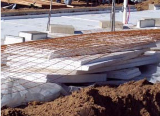
Styrofoam and wire mesh form the substrate for anchoring the radiant heating tubes in place
