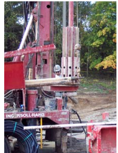
Nineteen geothermal wells are drilled 220 feet into the ground; each takes about half a day to drill
