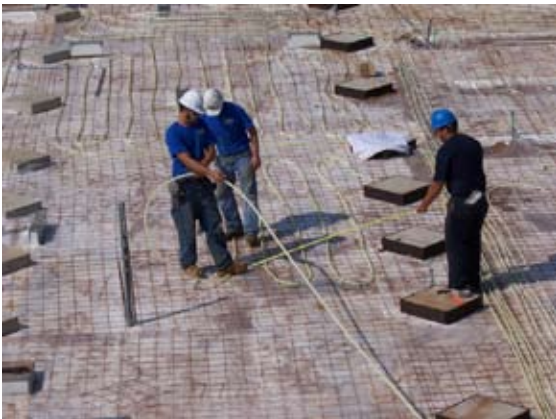
Workers install over 8,400 linear feet of plastic tubing for radiant floor heating in the display area, library and offices
