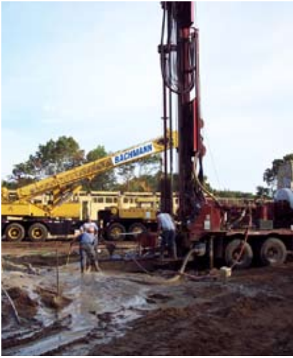
A team controls the flow of slurry – mud and water – extracted from the well as the drill goes deeper into the ground
