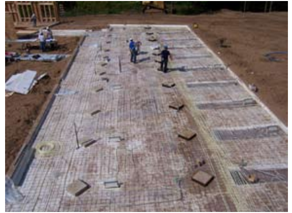
Tubing being installed in the area that will become Aldo Leopold Foundation staff offices
