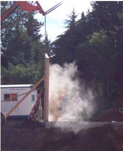
A crane holds the wall in place while workers drill screws into the concrete pad to anchor the base
