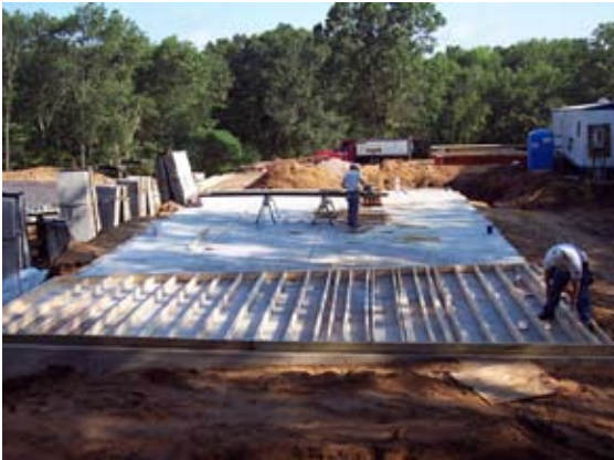
Workers cut studs to length and nail them in place to form the structure of the wall
