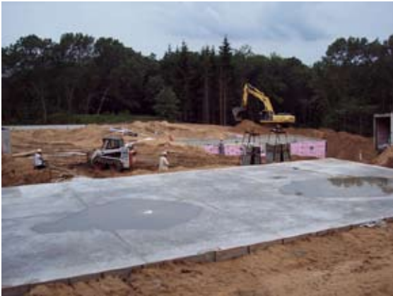
This concrete pad will form the floor of the Axe-in-Hand Stewardship Workshop
