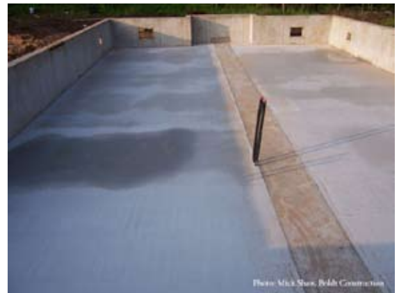
This completed sub floor will be under the finished wood floor in the meeting hall in the new Legacy Center
